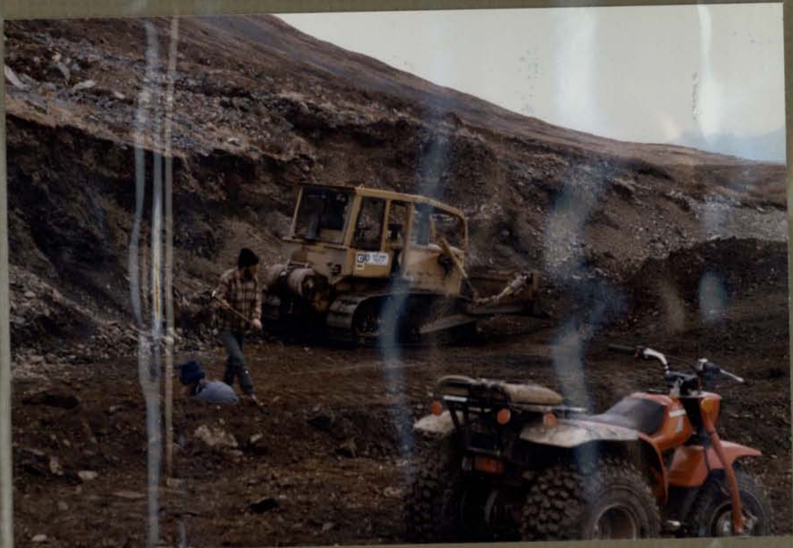
Deepening Trench #1 in October. The floor of the trench is rhyolite—in part gold-bearing. The wall is slumped argillite.
