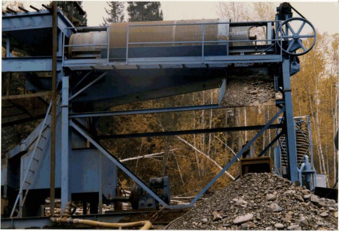
FREGOLD'S TROMMEL PLANT, STOCK PILING GRAVEL COBBLE FOR CONSTRUCTION OF SETTLING PONDS
