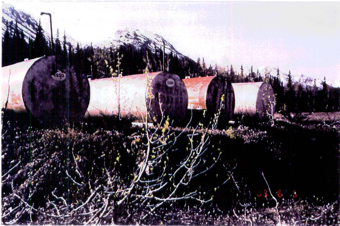
REAR VIEW OF 10,000 GALLON TANKS
