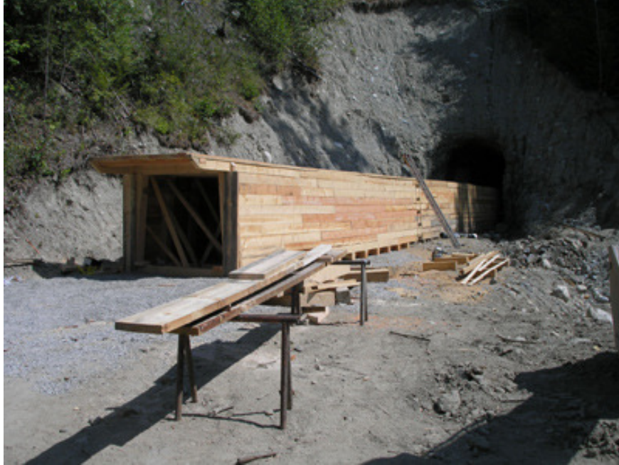
The adit construction completed with 37 sets on 3' centers, covered with 3" x 8" planking ready to be buried. The interior is cross-braced to prevent movement while being filled.
