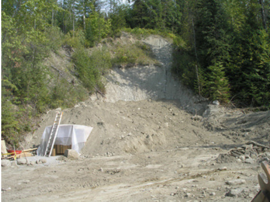
Tuesday August 22, 2006 Backfilling is complete and ready for inspection. The yard was cleared of backfill and leveled.
