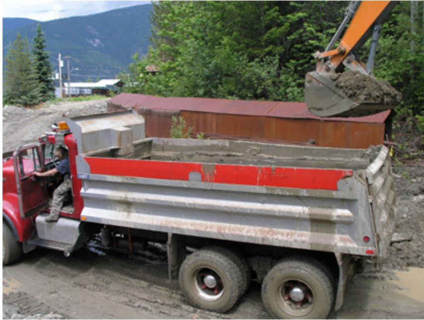
A 10 ton tandem dump truck from W.W. Excavating arrived at noon to augment the digging
