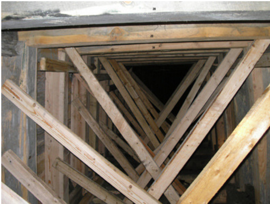
All the sets were photographed to check for any movement by backfilling
