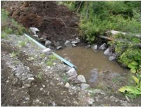
Stream Inlet Sediment Trap and Armoring
