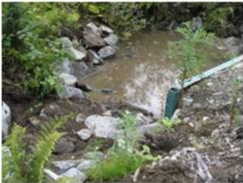
Stream Inlet Sediment Trap and Armoring
