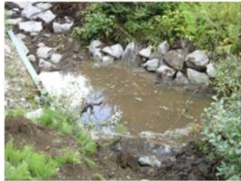
Stream Outlet Sediment Trap and Armoring
