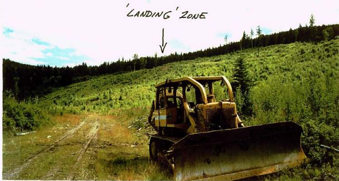
MEGATON: VIEW SOUTHEASTERLY. TD 20E DOZER PARKED IN FOREGROUND BY URSA MAJOR ROAD
