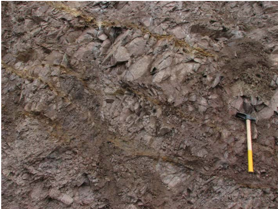
Figure C-8. Outcrop 66. Paramount zone. Intense fracturing and faulting of granodiorite. Note sub-parallel fault gouge trending north east and dipping 40-degrees.
