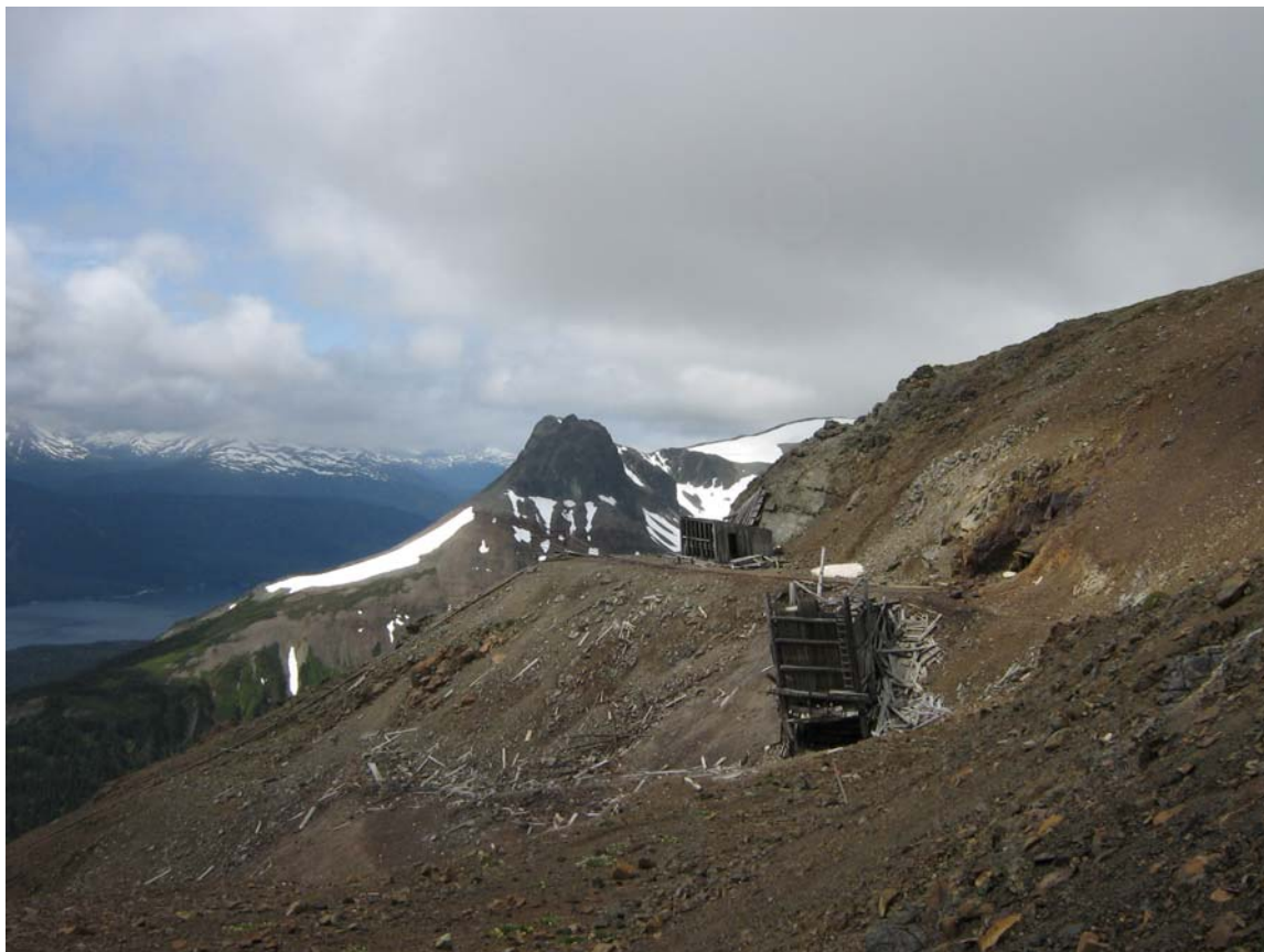
Photograph 1: View of 6400 level adit with partially collapsed ore bin in the foreground, and Rhine Crag and Tahtsa Reach in the background.
