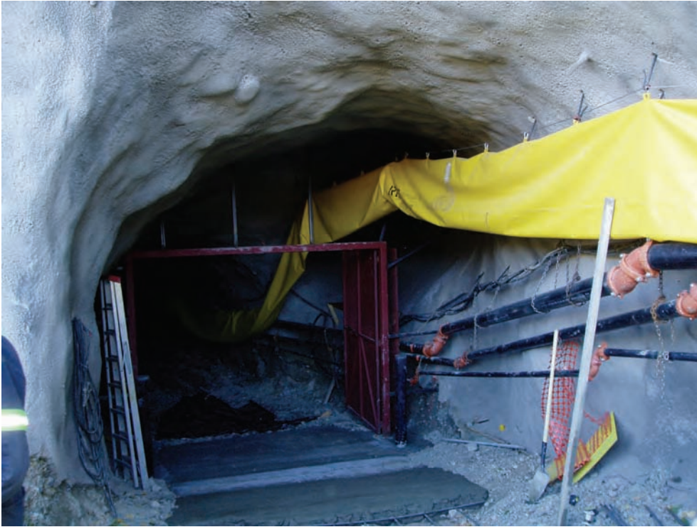
Top Left: Portal showing ventilation and electrical
