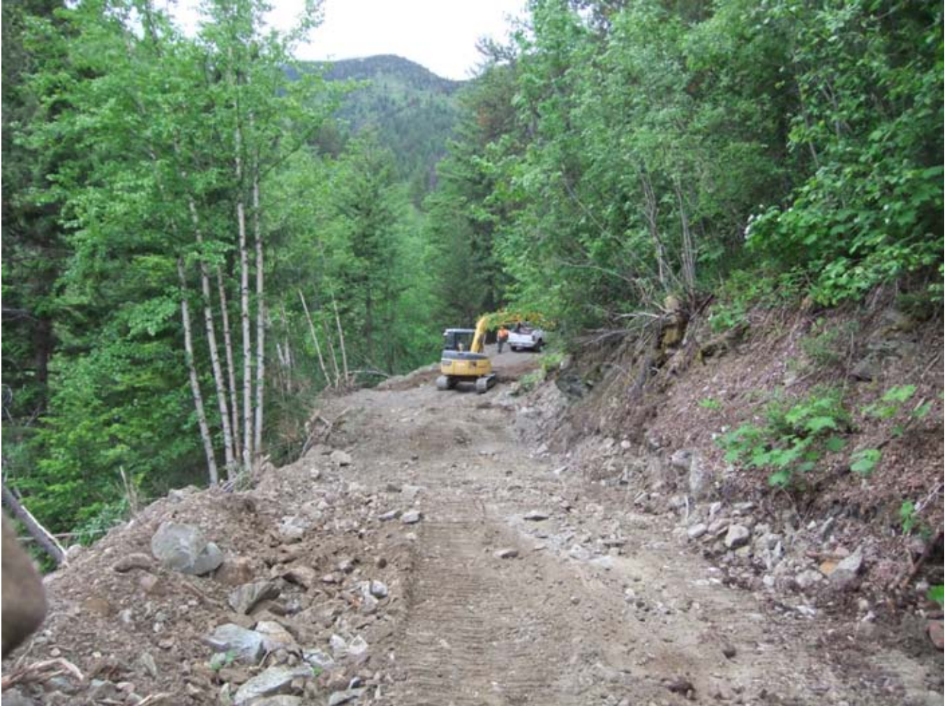
Photo 4: Finalizing the last portion of the road along the eastern slope across from the DOT Zone – early June, 2011.
