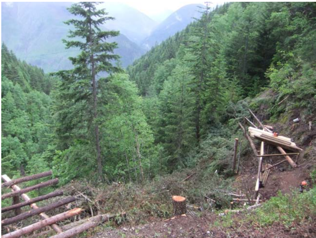
Photo 6: Constructing drill pad 2 (photo below), to the left of photo emergency helipad. Looking southerly down slope to the Nahatlatch River valley.
