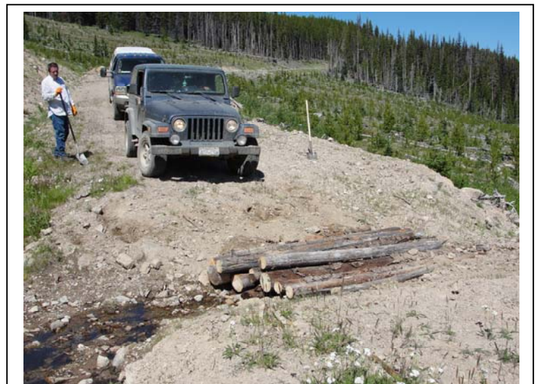
Photo 2: Remediating access road to the south part of the Property. Photo by Craig Lynes, Rich River Exploration, 14 August 2011.
