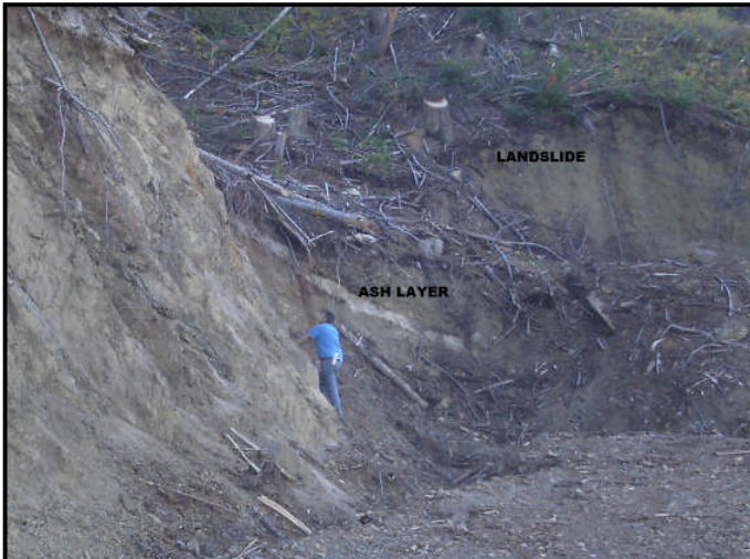
Photo 2 Picture of Landslide and Ash Layer in Road Cut
