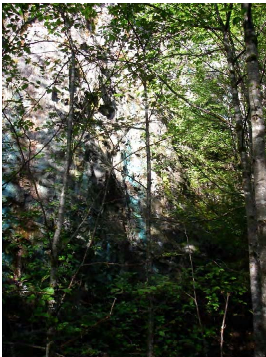
Photograph 6: Copper rich precipitate has formed on bedrock face where seepage is occurring. This is located on rock face above access road up to Pit No. 1.
