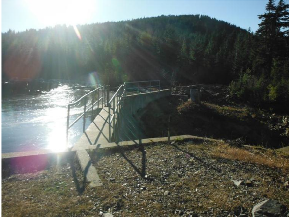
Photo B-11. A view of the concrete dam structure located at the north end of Holyoak Lake, on November 14, 2014.
