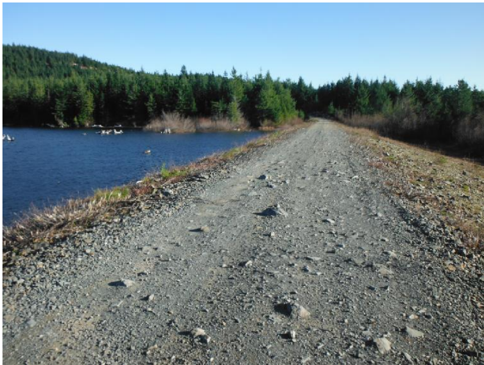
Photo B-10. A view of the earthen dam, located at the south end of Holyoak Lake looking south on November 14, 2014.
