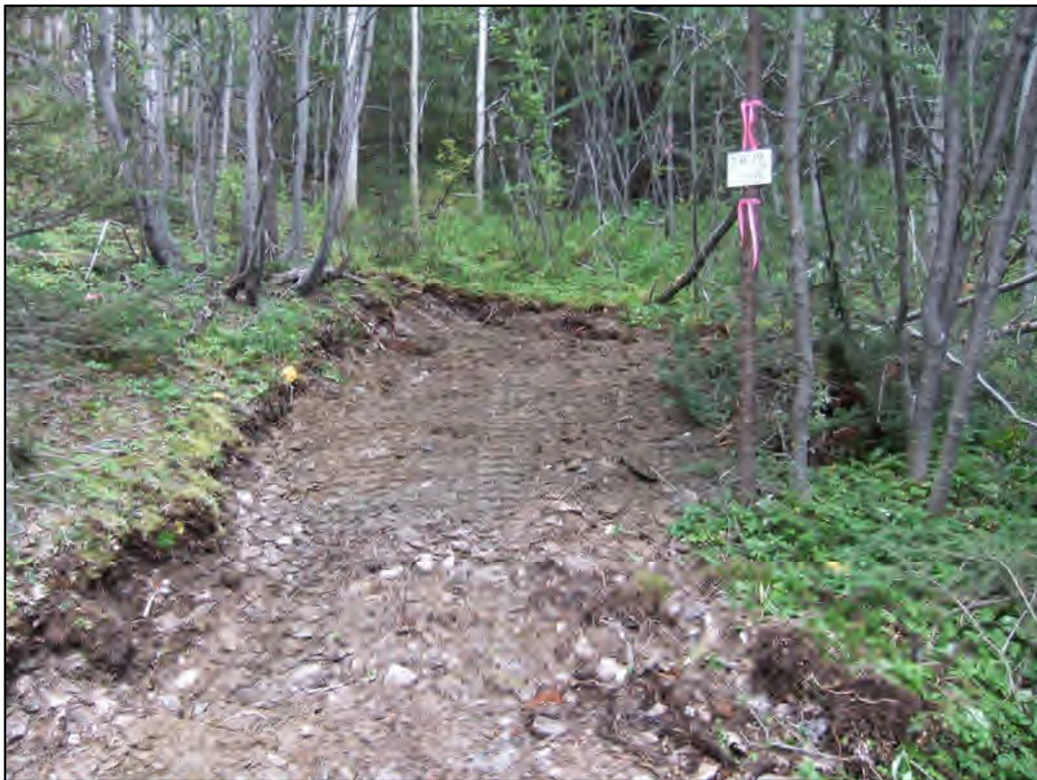
TR19/15, Filled In, Trench Marked with a Pink Ribbon on a tree with a Labelled White Board
