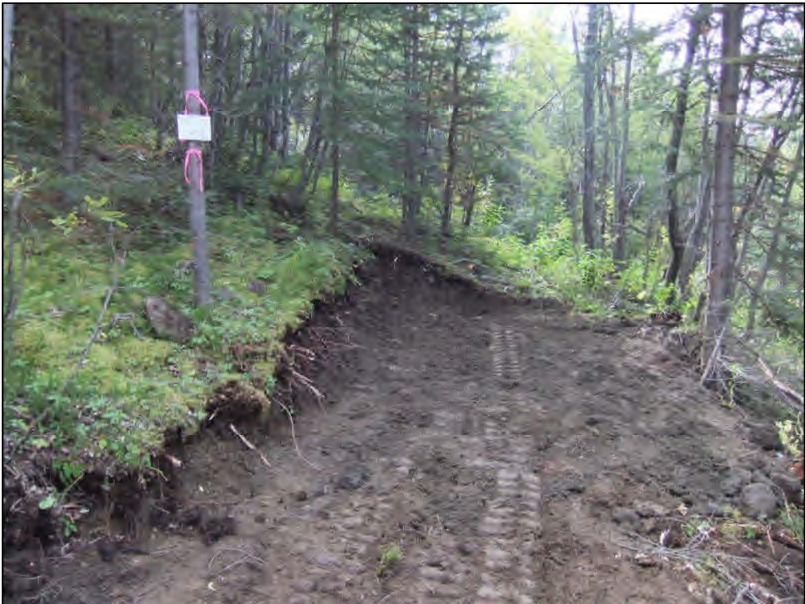
TR20/15, Filled In, Trench Marked with a Pink Ribbon on a tree with a Labelled White Board
