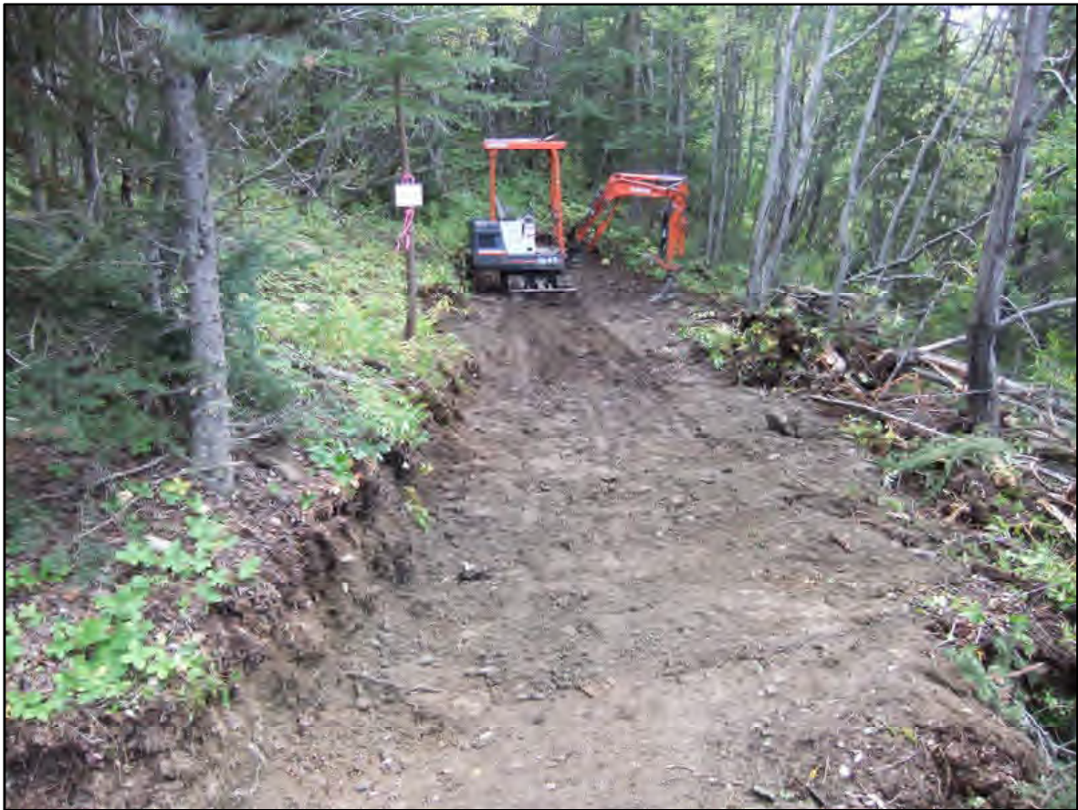
TR21/15, Filled In, Trench Marked with a Pink Ribbon on a tree with a Labelled White Board
