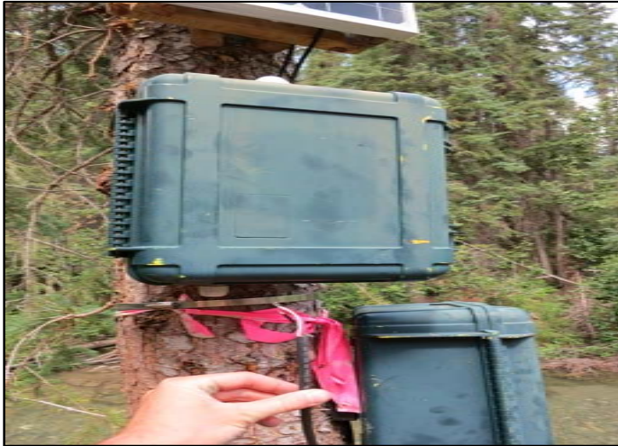
PHOTO 9 H5 Hydrology Site - Animal damage, July 2015
