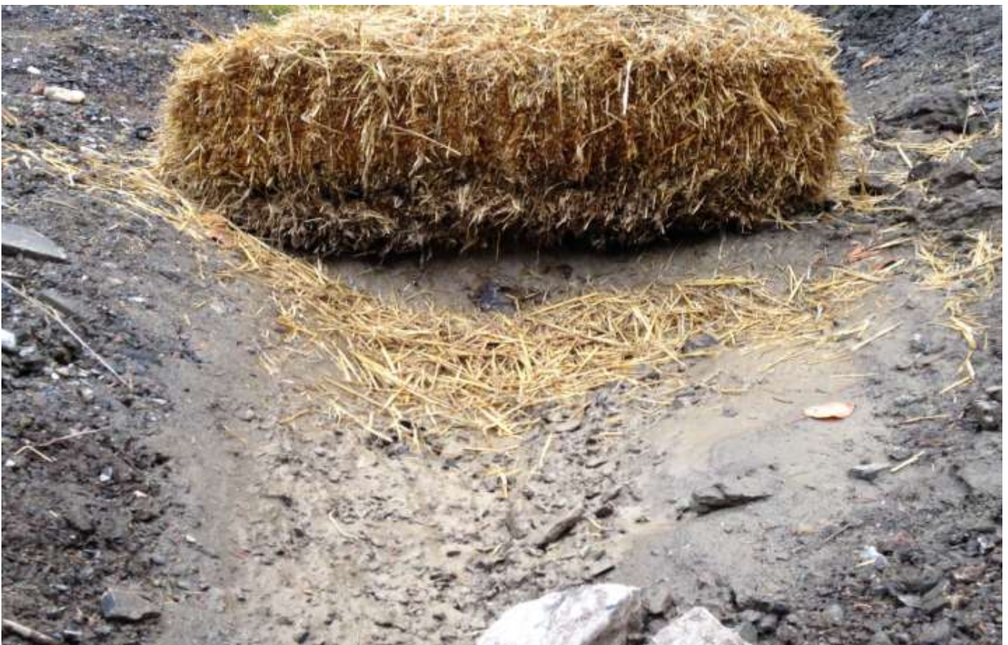
Replaced Ditch Block that worked well during excessive rain as you can see the high water mark were water was filtered (After)
