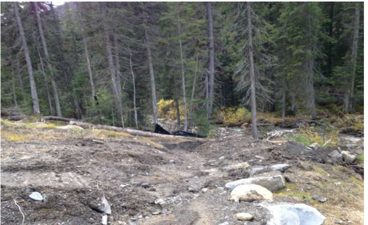
Large Catch Basin above creek (After)
