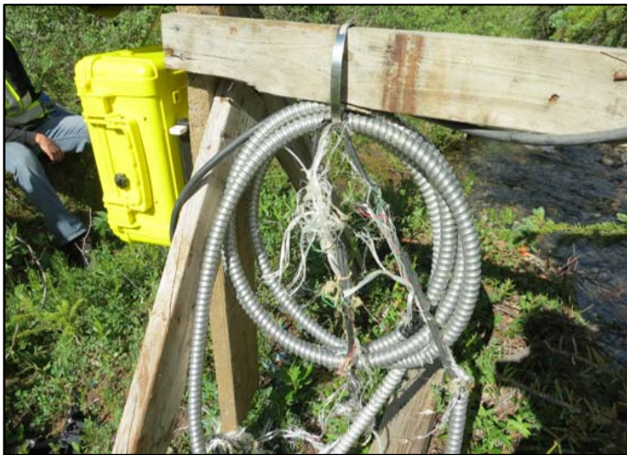
PHOTO 11 H7 - Hydrology Site - Animal damage, July 2015
