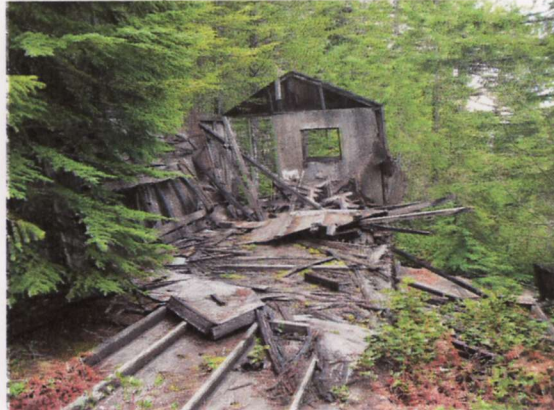
another collapsed cabin, near Sharon adit
