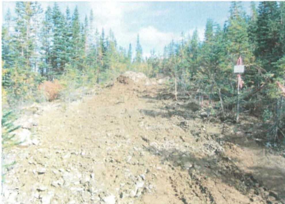
Figure 12 Exploration trench #TR25/16 marked and an estimated 8.2m filled. Roughly 4m remained unfilled and the far end of trench. Investigation of the remaining 4m will be scheduled for summer, 2017.
