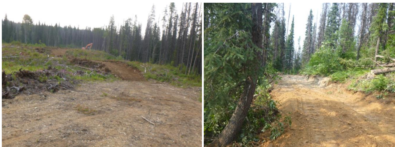
Figure 10 Photographs exploration access. Left: Excavated access trail starting from a logging landing within a cut block. Right: Excavated access trail through forested area.
