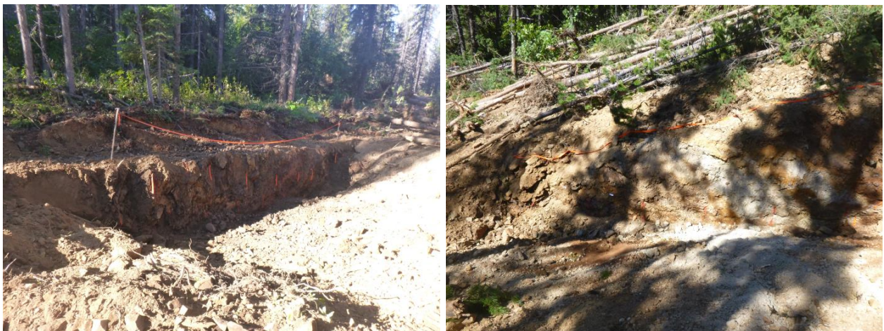
Figure 24. Photographs trench areas left un-reclaimed. Left: Mineralized zone in Trench 2 left exposed. Right: Mineralized zone in Trench 6 left exposed.
