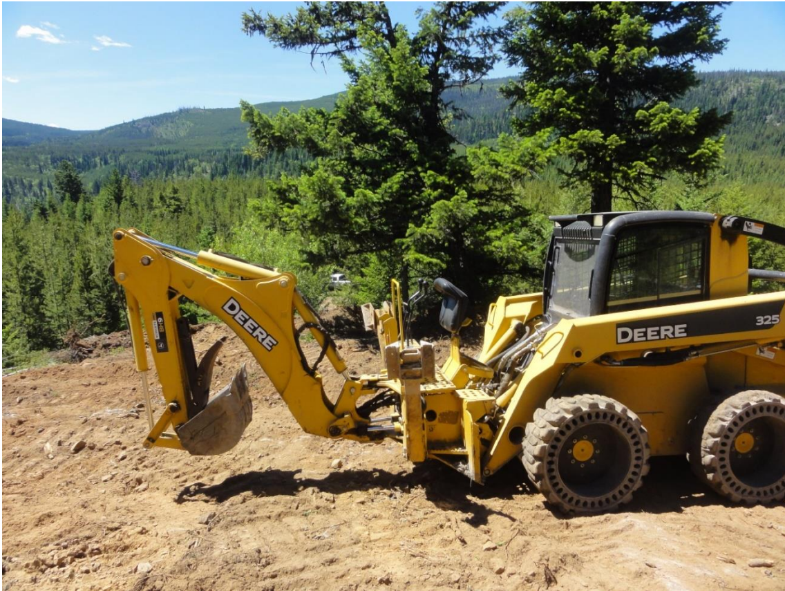
2010 JD 325 with backhoe attachment used for reclamation and operating 20 lb hydraulic chipping hammer for hand trenching and rock sampling/testing.
