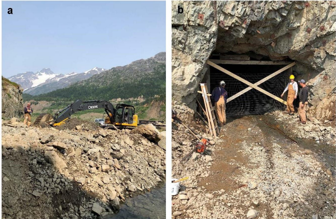
Figure 13: Photos showing reclamation work at portal D that includes (a) cleaning out of rock rubble and (b) reframing the adit and screening it off with wire.
