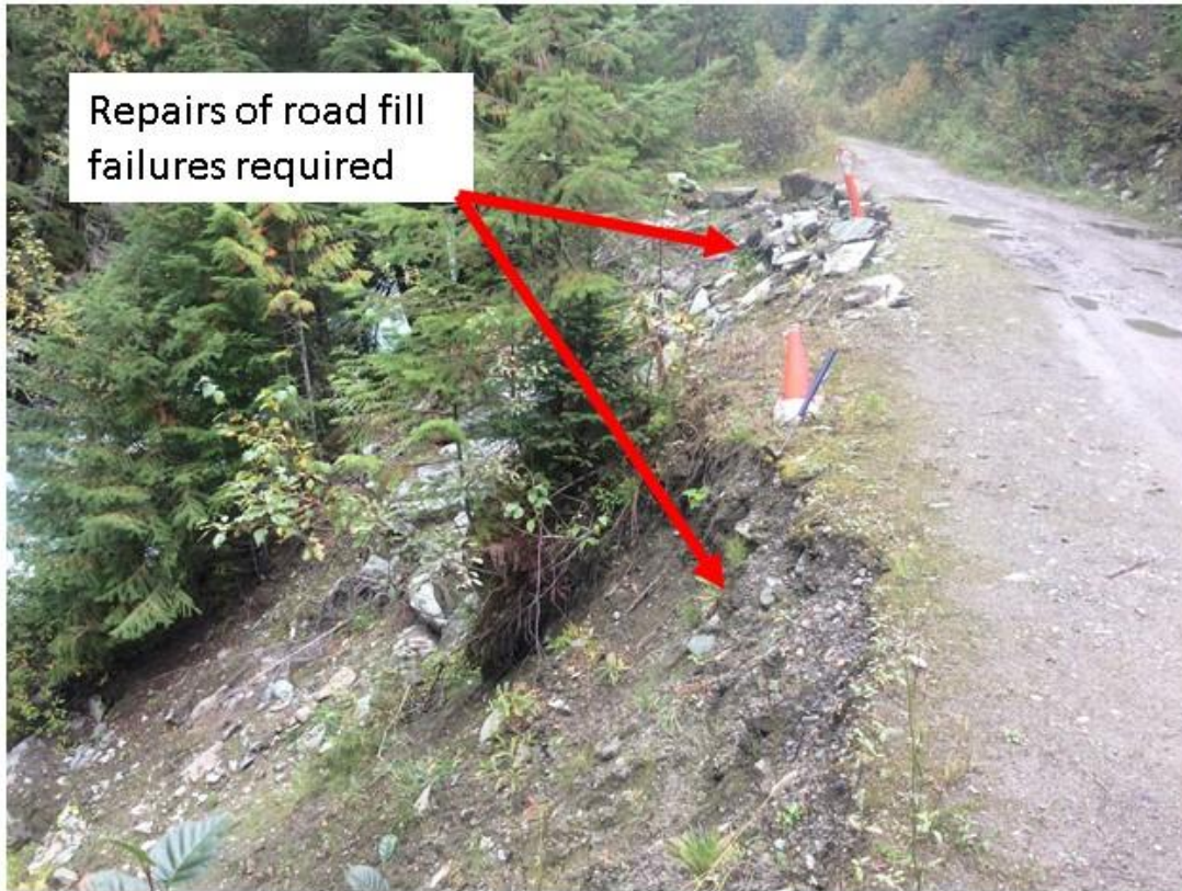
Figure 5: Fill Slope Repair Required. This is at the site where the vehicle was recovered.
