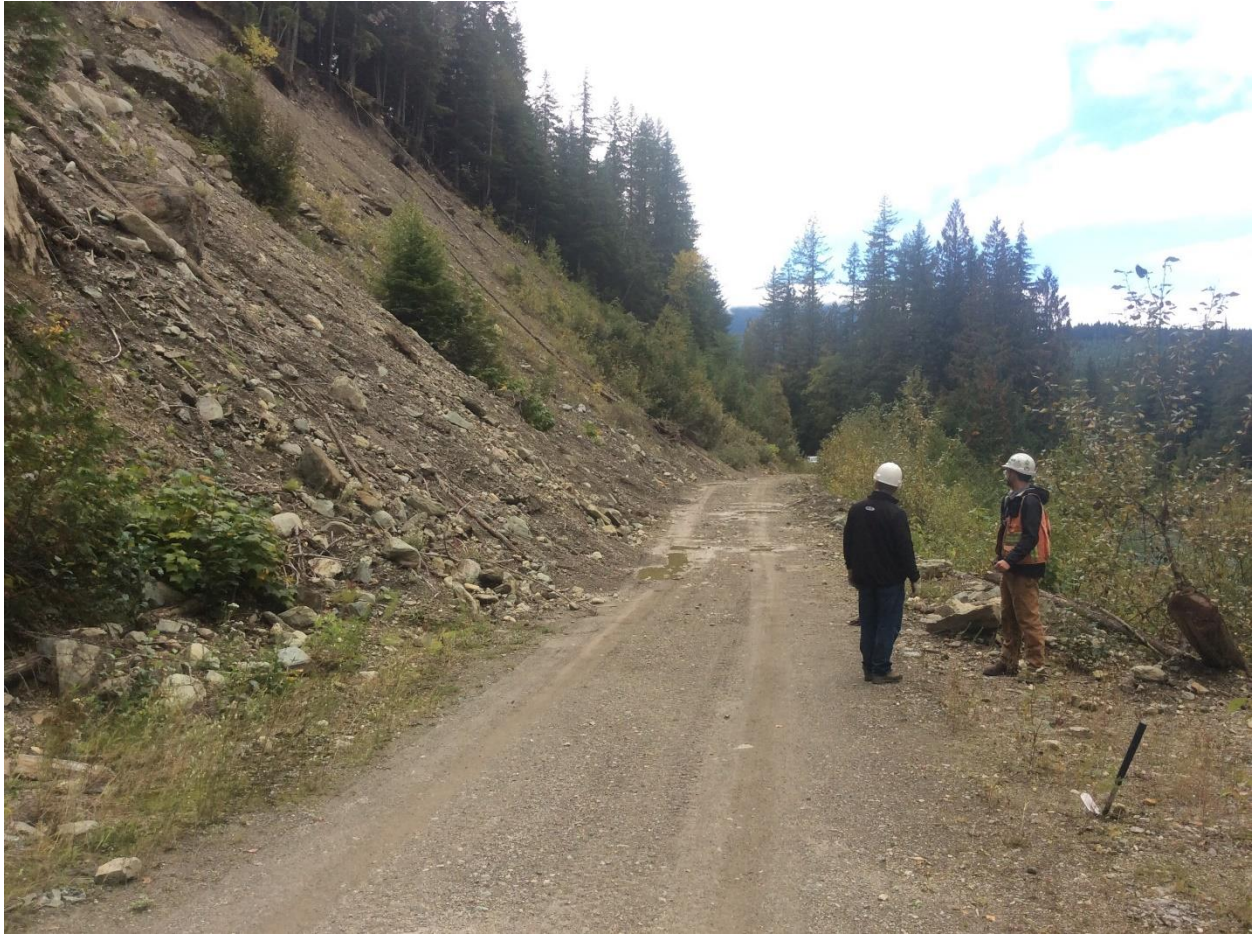
Figure 3: Raveling Slope. Note large boulders and debris on slope.
