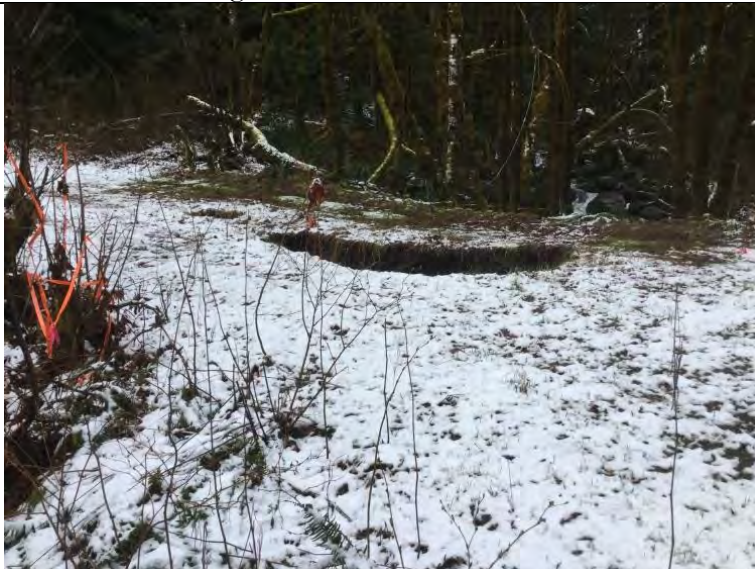
Photo 7 – Large hole in bridge across tributary of Seven Mile Ck.
