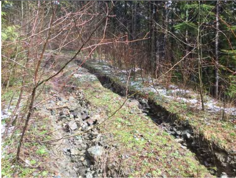
Photo 9 – Surface erosion of road from blocked drainage.
