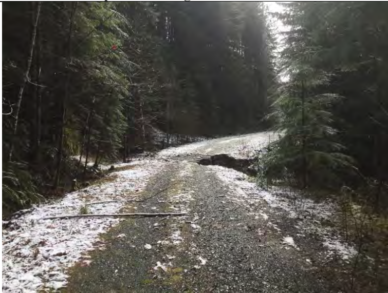
Photo 3 – Fillslope failure removing outer 1/2 of road surface.
