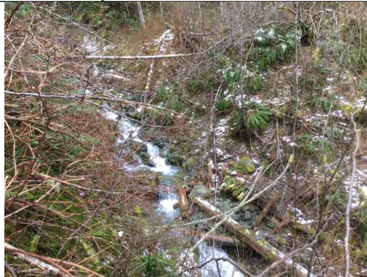
Photo 12 – Bridge removed from 15-20 m span of gully crossing on large tributary stream.
