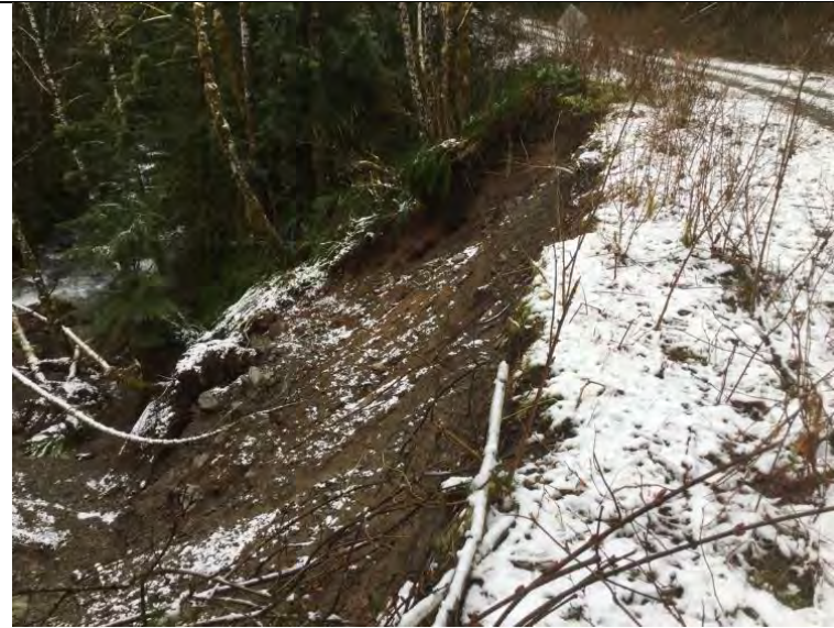
Photo 6 – Fillslope failure with tension cracks on outer 1/4 of road.
