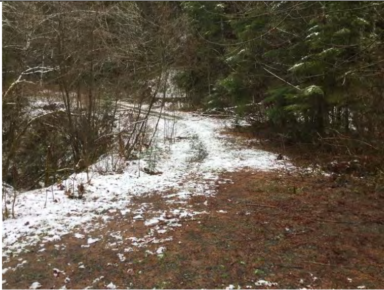
Photo 5 – Seven Mile Creek bridge partially rotten/failing on left side of crossing.
