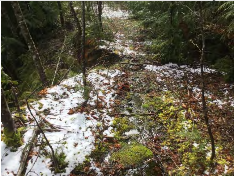
Photo 11 – Fillslope failure near blocked drainage.
